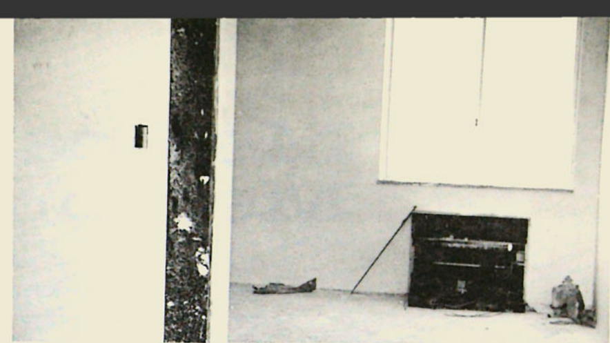
PATIENT ROOMS IN THE EXTENDED CARE FACILITY WILL BE MOSTLY DOUBLE ACCOMMODATIONS. AT THE LEFT IS THE EXTRA-WIDE BATHROOM DOOR, MADE TO ACCOMMODATE A WHEELCHAIR EASILY. ALL ROOMS WILL BE AIR CONDITIONED, WELL LIGHTED, AND BRIGHTLY DECORATED. THERE WILL BE 50 PATIENT BEDS ON EACH FLOOR.
