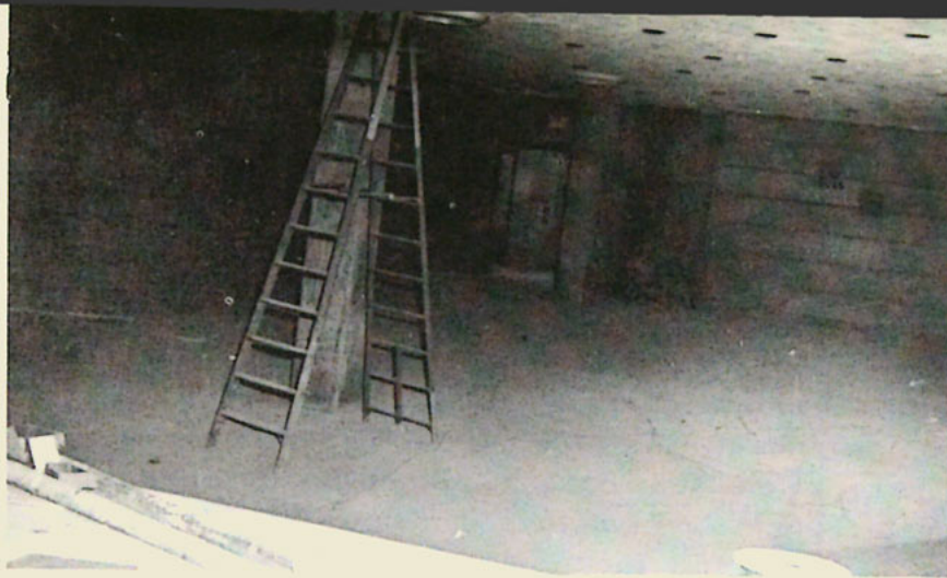
THE 186-SEAT AUDITORIUM ON THE LOWER LEVEL, SHOWN ABOVE FROM THE STAGE, WILL BE DECORATED WITH BRICK WALLS, CARPET, MODERN SEATS, AND RECESSED LIGHTING. THE AUDITORIUM PROJECTION BOOTH CAN BE SEEN AT CENTER RIGHT.
