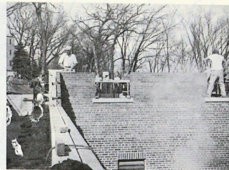
By November 15, the masonry on the laundry is expected to be finished.
