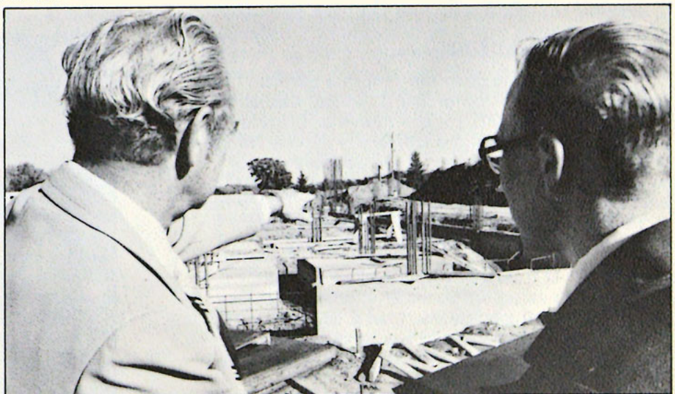
Construction of Saint Benedict's Center began almost immediately after its ground-breaking ceremonies held September 9, 1976. Dale Stein, Assistant Administrator for Shared Services, is pictured above right with Al Fischer, Project Architect, reviewing the progress made during the first few weeks of construction.
