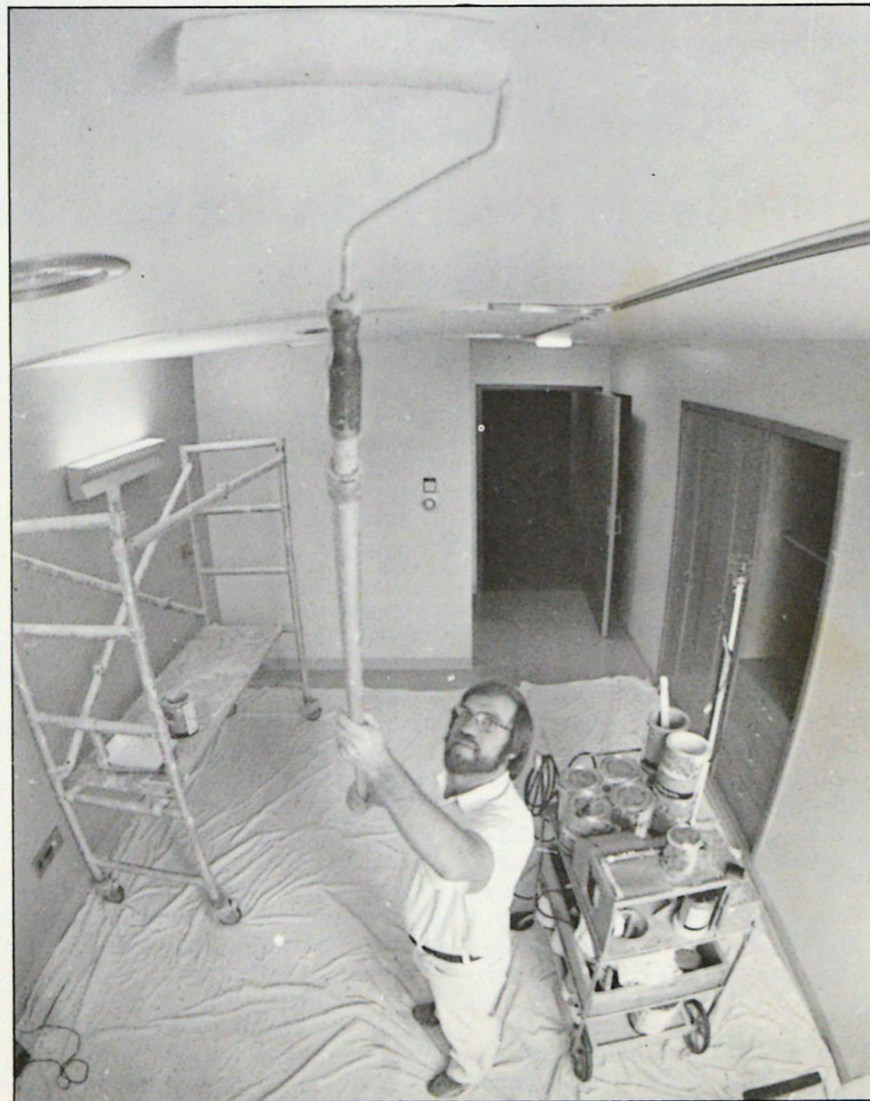
Tom Schreifels, painter, right, adds fresh paint to five rooms on 3 Northwest which will be used as the MHU's Interim Satellite Unit.
