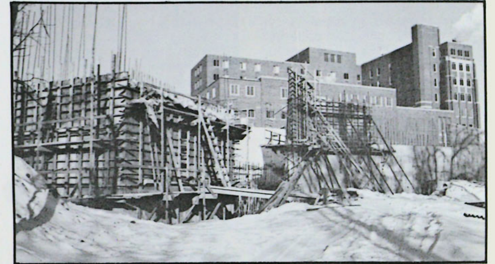
Work continues on the Southeast construction site. Workers are now building the elevator and stair tower
